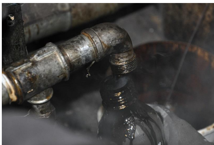
Figure 5 – Oil sampling from condenser 1
